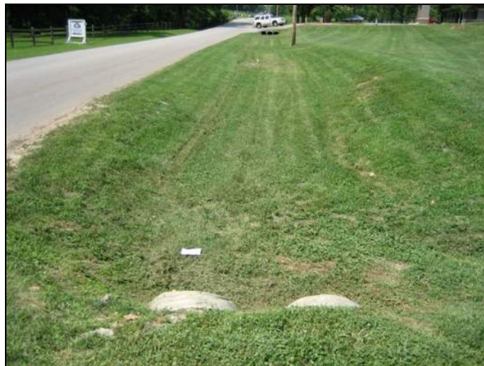
Photograph WQ-9 – Example of a Grass Swale.
