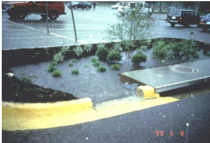
Photograph WQ-4 – Example of Porous Landscape Detention.
