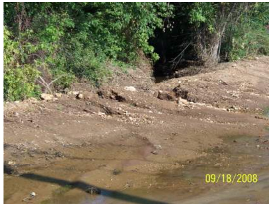
Photograph CS-1 – Example of Erosion during Construction
