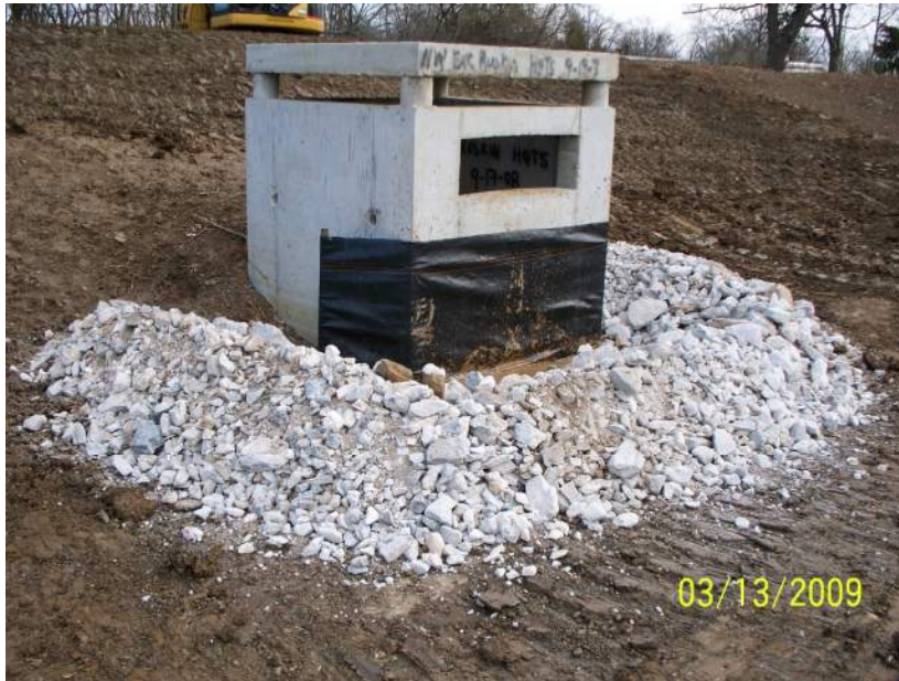
Photograph CS-5 – Example of Inlet Protection
