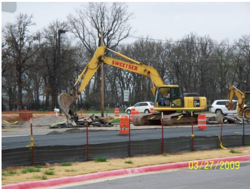
Photograph CS-4 – Example of Silt Fencing
